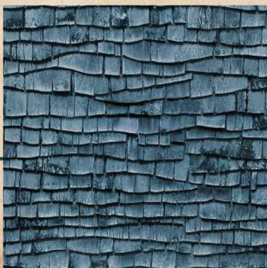
Broken Wooden Shingles
